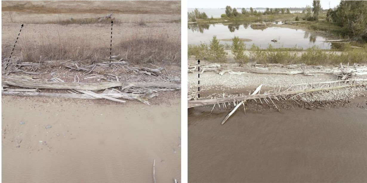
Figure 58. These are oblique drone images between Pilings F and G. The left photo is during lake draw down 2023 and the right photo from same area in August 2023. The black dotted arrows show flow paths from wave overwash.
